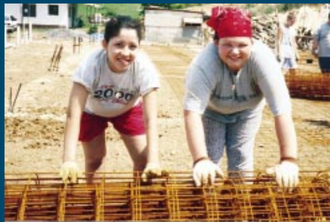
At work — Summer Chavis and Nichole Winter roll out wire in preparation for pouring concrete
