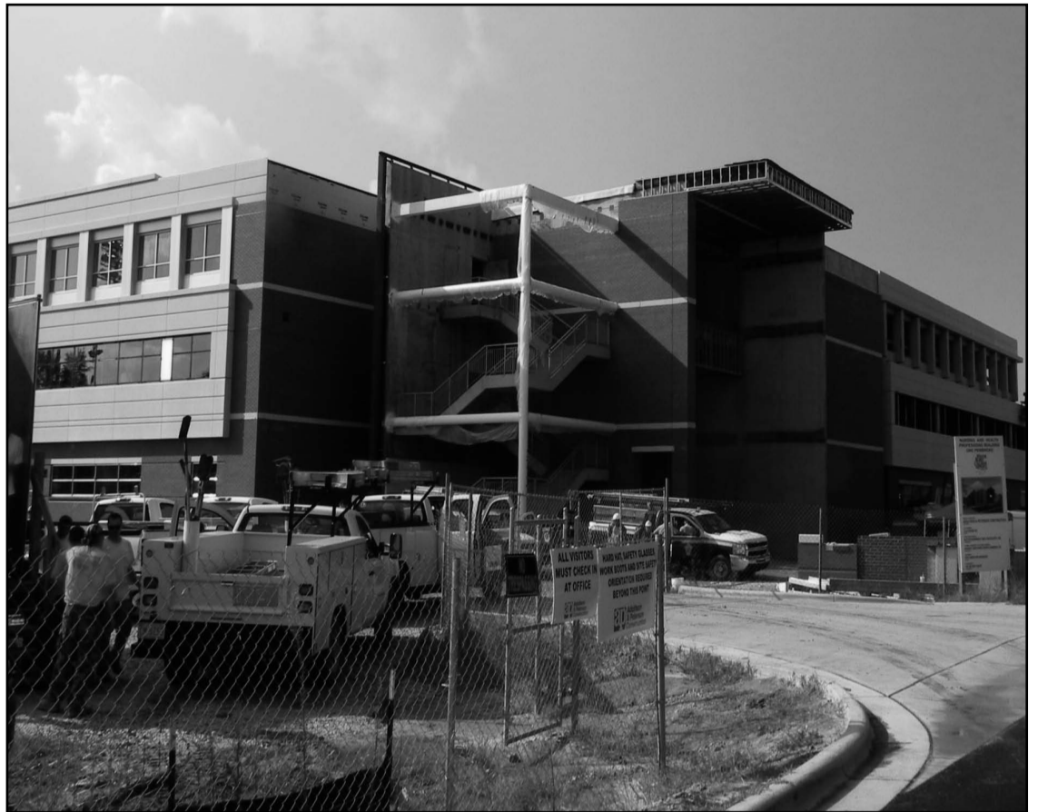
Construction on the new Nursing Health Professions Facility has been going on for nine months. The 87,000 square foot facility is set to open in January 2012 in time for the spring semester. The social work department will join the nursing department in the new building. Photo by Mindy Hubbard
