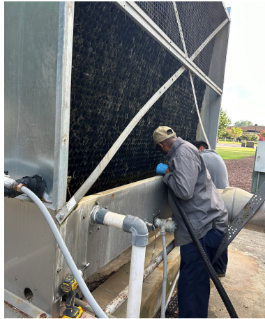
GPAC – cooling tower cleaning
